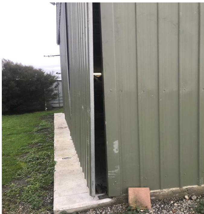
The big shed door off its tracks
