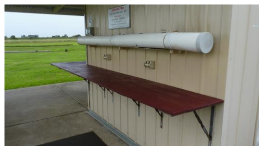
Western Charging station cleaned up, after LiPO fire damage
